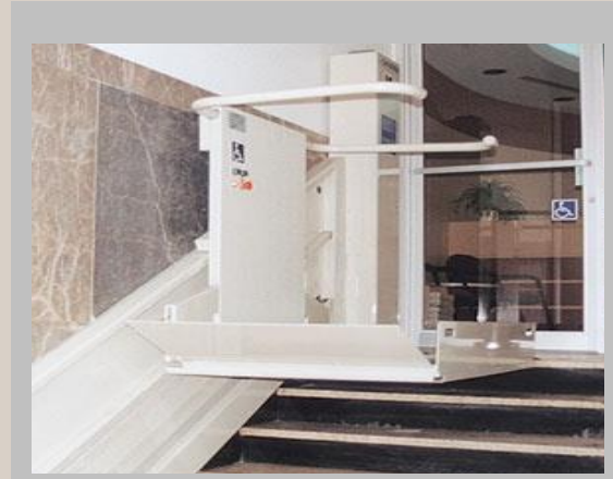
A stairlift of the type shown which requires inspection under legislation every 6 months
