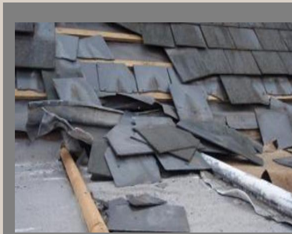
A church roof which has had some lead stolen – with considerable additional damage to the surrounding slates.
