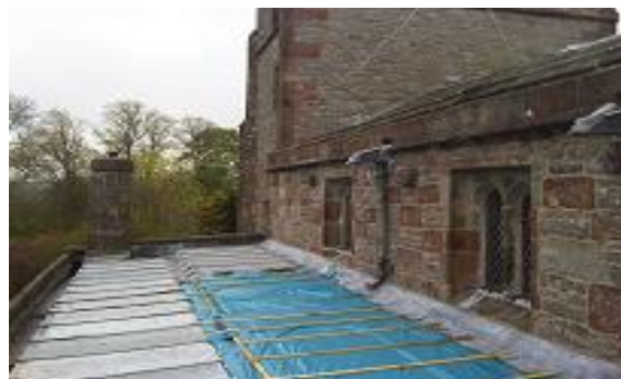
A church stripped of some of its lead; almost 150 incidents of this type have been reported to us in the last 2 years by Church of Scotland congregations.
