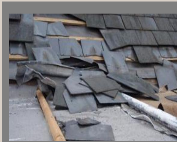
A church roof which has had some lead stolen – with considerable additional damage to the surrounding slates.
