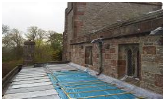
A church stripped of some of its lead; almost 150 incidents of this type have been reported to us in the last 2 years by Church of Scotland congregations.
